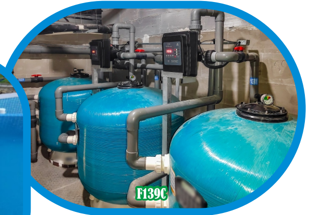
▲山东某泳池公司过滤设备 Shandong Pool Company Filtration Equipment
